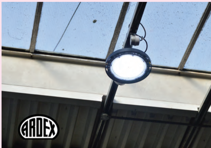
BAL LED lighting has been installed across the UK group
